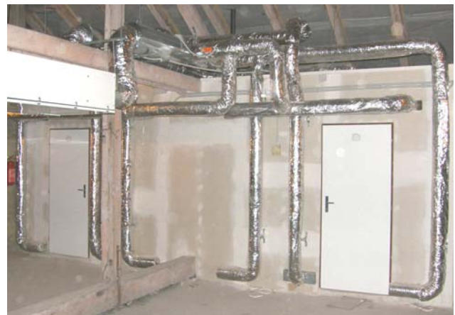
Pict. 2. Controlled ventilation system
